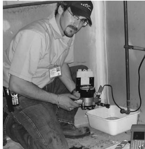
NEPTUNE'S PROJECT MANAGER, DAVID ONER, INSTALLING A T-10 METER WITH R900 MODULE IN BRANDON.
